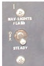
Nav Lights Switch
