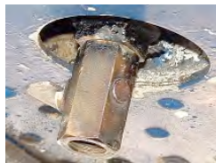
Aux Tank Drain
